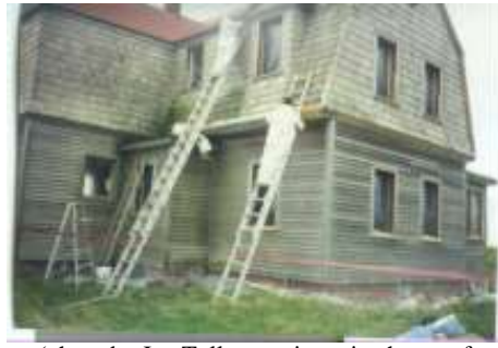
(photo by Joe Tully - engineer in charge of the Coast Guard's 1994 restoration of the lighthouse)
